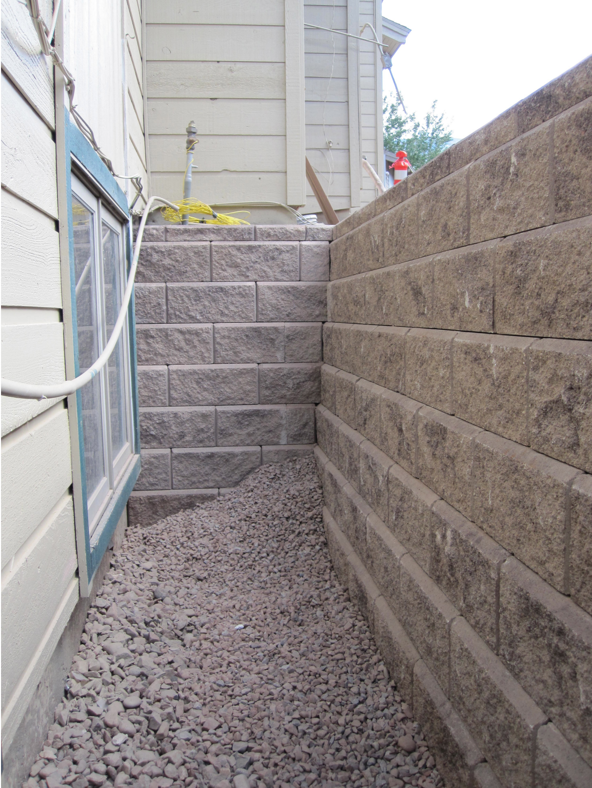
The final two pictures show the new color palette on the upper buildings and the almost completed stairways with new concrete treads, new iron balusters, and new Brazilian wood landing. Still to be installed is the handrail on the wood side railing.
